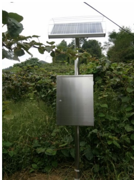
Figure 8. The picture of hardware physical 图 8. 安装好的硬件实物图
