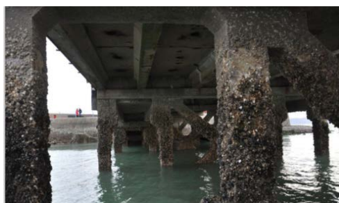
Figure 1. Marine mollusk animal attachment and corrosion damage to marine engineering structures
