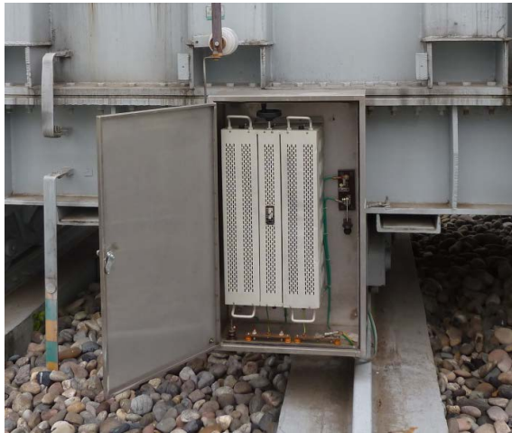
Figure 7. Core grounding current limiting resistor 图 7. 铁芯接地限流电阻
