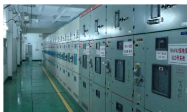
Figure 9. The overall environment of the high pressure chamber at the substation 图 9. 变电站高压室整体环境
