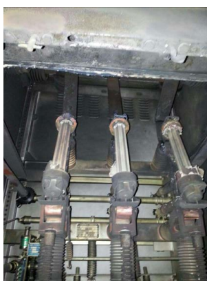
Figure 8. Situation of power distribution station 图 8. 配电站故障情况
