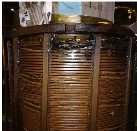
Figure 3. Main transformer high voltage fault instability coil 图 3. 主变高压故障失稳线圈
