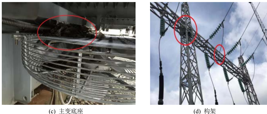
Figure 7. Location and structure of bird damage 图 7. 鸟害发生位置结构
