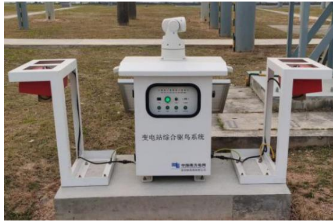
Figure 8. Integrated bird repellent system 图 8. 综合驱鸟系统
