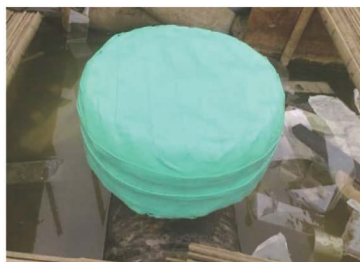
Figure 1. The application of viscoelastic body in overall sealing of flanges, bolts and nuts 图 1. 利用黏弹体对法兰及螺栓螺母进行整体密封防腐
