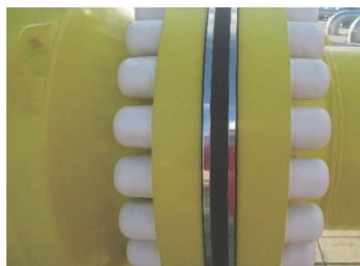
Figure 2. The application of plastic cap in sealing the nuts 图 2. 利用塑性保护帽对螺母进行密封
