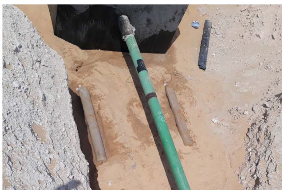
Figure 18. Cathodic protection installation 图 18. 阴极保护安装
