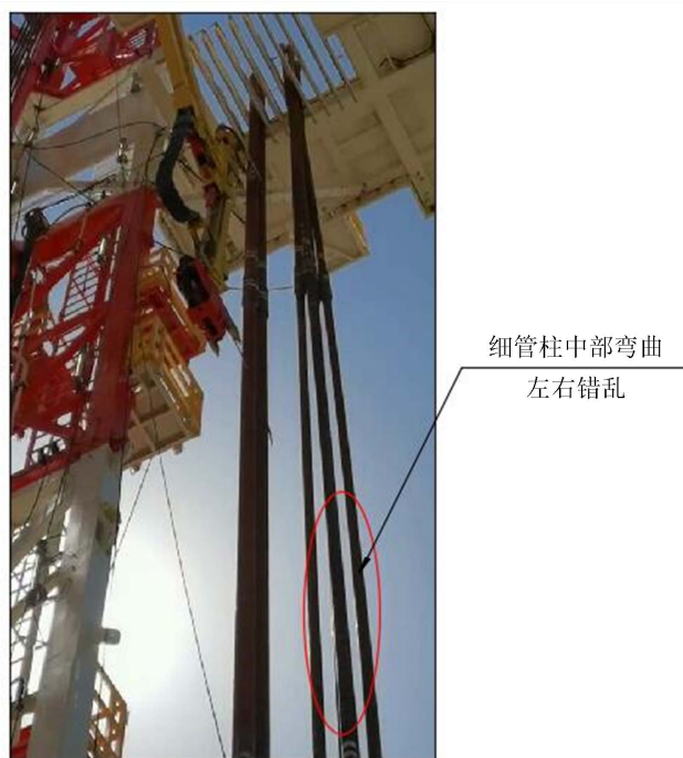
Figure 1. Physical picture of pipe string riser bent in the middle and disordered from left to right during pipe laying operation
