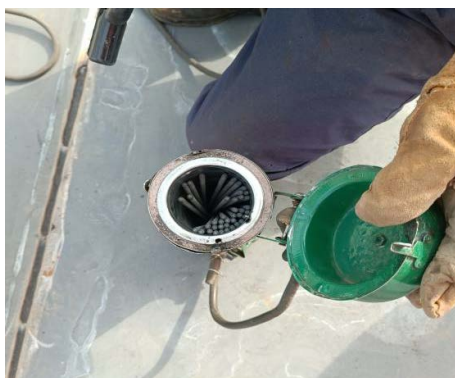
Figure 1. Failure of insulation barrel
