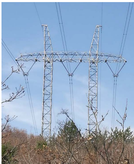
Figure 1. Tower of 330 kV high voltage power transmission line in Sipan District of Yuhua Coal Mine
