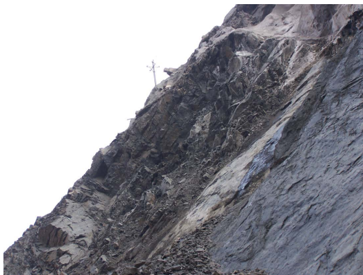
Figure 2. Collapse failure of bench slope 图 2. 台阶破崩塌破坏
