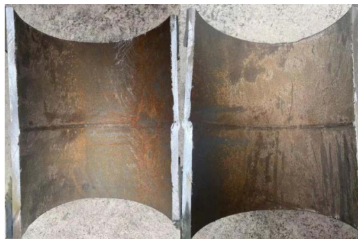
Figure 4. The macroscopic feature of the corrosion gas tubulation's wall inside
