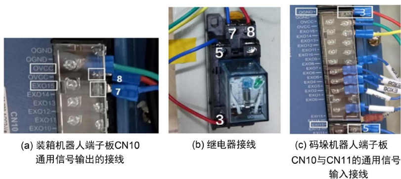
Figure 7. Enlarged wiring diagram of control system of packing manipulator 图 7. 装箱机器人控制系统接线实物放大图
