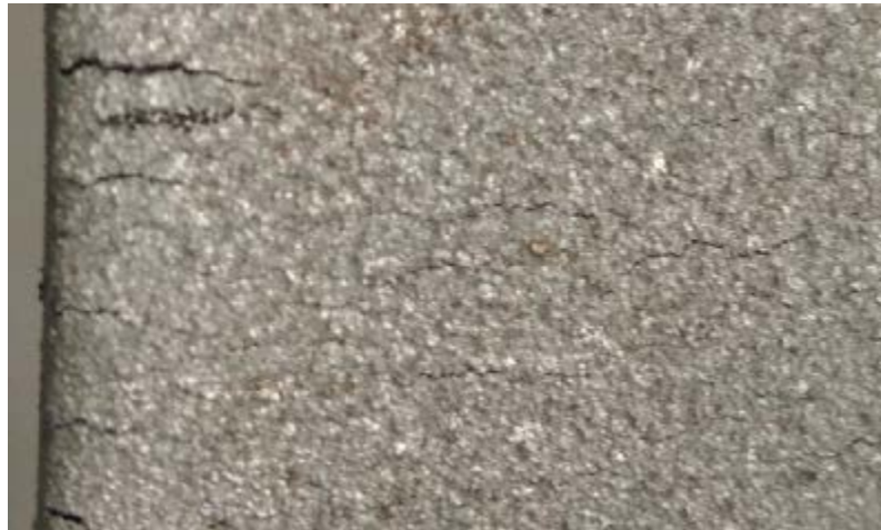
Figure 10. Bending specimen 2 cracking state 图 10. 弯曲试样 2 开裂状态
