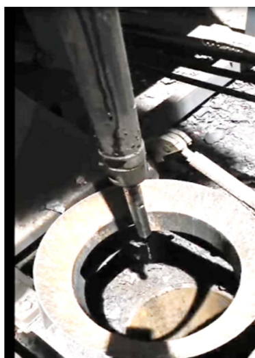
Figure 3. Water leakage of sub lance
