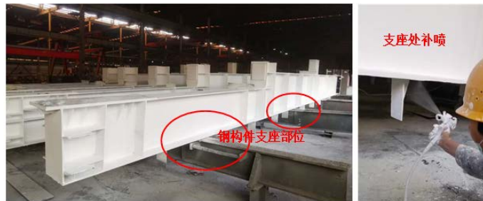
Figure 6. Re-spraying fireproof coating on hidden parts of steel components 图 6. 钢构件隐蔽部位补喷防火涂料
