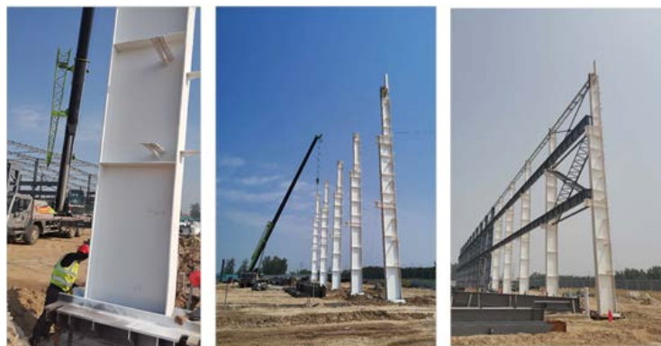
Figure 7. On-site assembly of steel components with pre-painted fireproof coating 图 7. 预涂装钢结构防火涂料构件现场装配化施工
