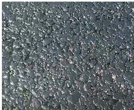
Figure 5. Spraying high performance trackless emulsified asphalt on the newly paved middle course 图 5. 新铺中面层上喷洒高性能不粘轮乳化沥青
