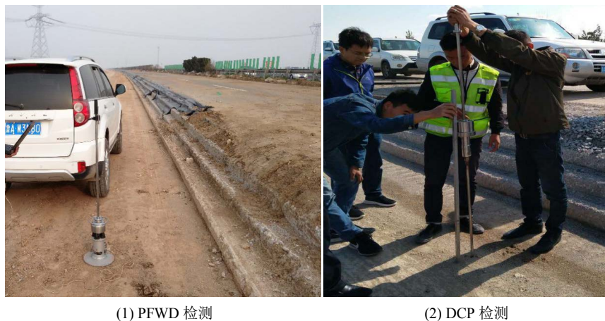
Figure 2. On-site inspection of the top surface of new and old road beds
