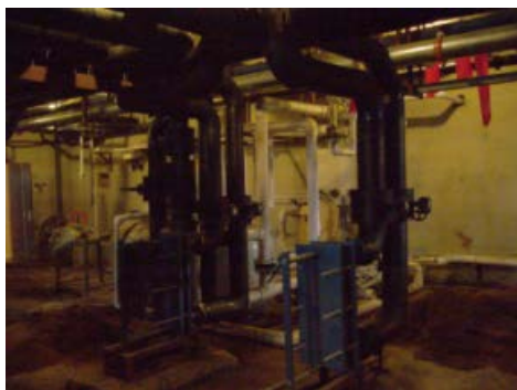
Figure 1. Air conditioning room real map
