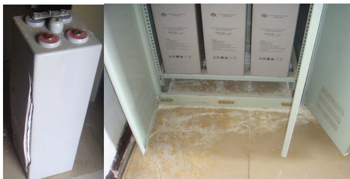
Figure 5. Battery frosted leading to leakage
