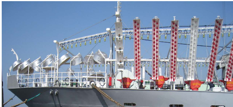
Figure 3. Installation result diagram of light box for saury 图 3. 秋刀鱼集鱼灯灯箱的安装效果图
