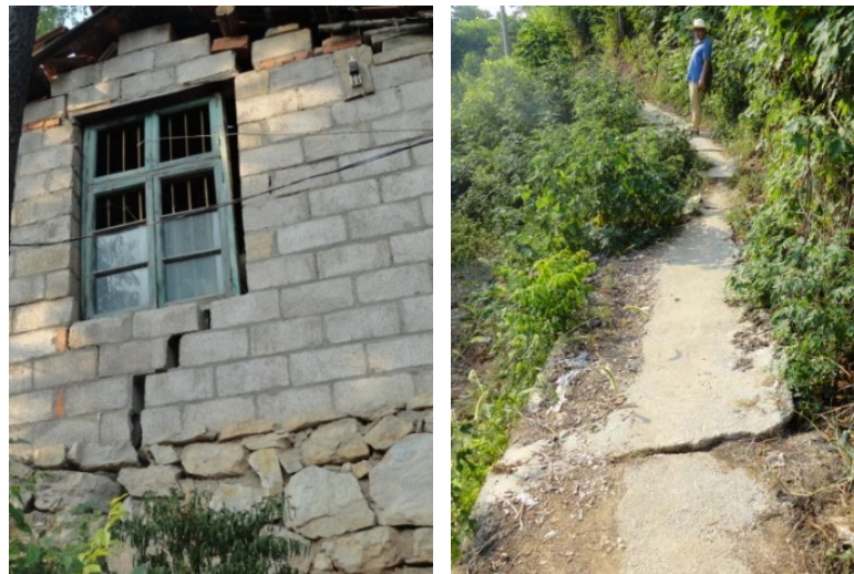
Figure 5. Deformation of buildings caused by landslides 图 5. 滑坡造成建筑物变形
