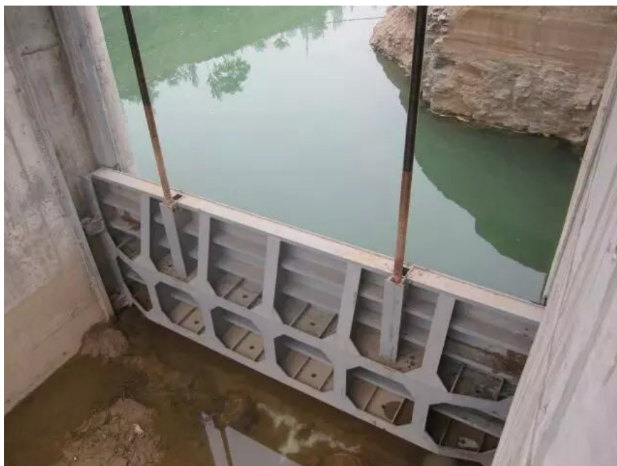
Figure 3. Deposit near the gate 图 3. 闸门淤积
