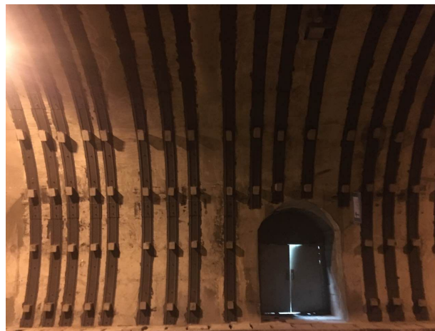
Figure 7. Construction effect of bolt + W steel strip support 图 7. 锚杆 + W 钢带支护施工效果图
