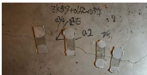
Figure 2. Slide monitoring cracking
