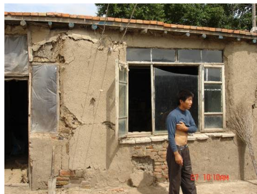
Figure 7. The horizontal cracks of masonry-mud-timber roof structure 图 7. 林甸地震中砖 - 土墙 - 木屋顶房门洞水平贯通缝
