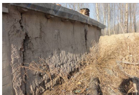
Figure 3. The vertical cracks of mud-timber roof structure 图 3. 前郭地震中的土坯 - 木屋顶结构竖向贯通缝
