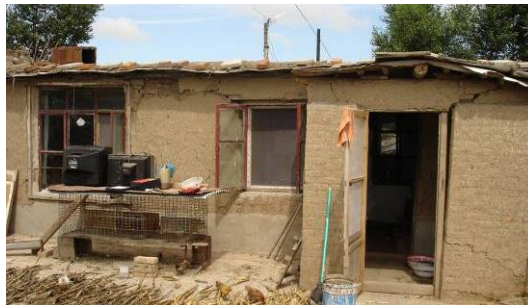
Figure 5. The diagonal cracks of masonry-mud structure 图 5. 林甸地震中砖 - 土墙 - 木屋顶房门洞斜裂缝
