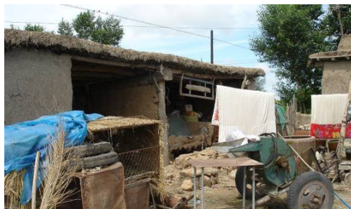
Figure 1. The collapse of mud house in Lindian earthquake 图 1. 林甸地震中的泥草房倒塌
