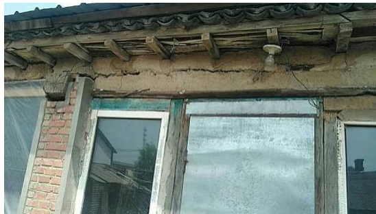
Figure 6. The horizontal cracks of masonry-mud-timber roof structure 图 6. 林甸地震中砖 - 土墙 - 木屋顶房门洞水平贯通缝
