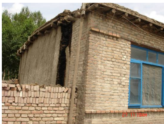
Figure 8. The roof collapse of masonry-mud-timber roof structure 图 8. 松原地震中砖 - 土墙 - 木屋顶房纵横墙脱落
