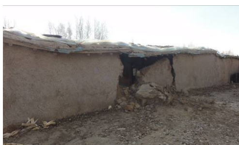
Figure 2. The collapse of mud house in Qianguo earthquake 图 2. 前郭地震中的泥坯房倒塌
