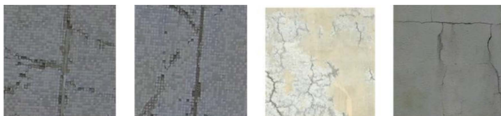
Figure 7. Four examples of cracks in exterior wall 图 7. 四个外墙(瓷砖)裂缝实例
