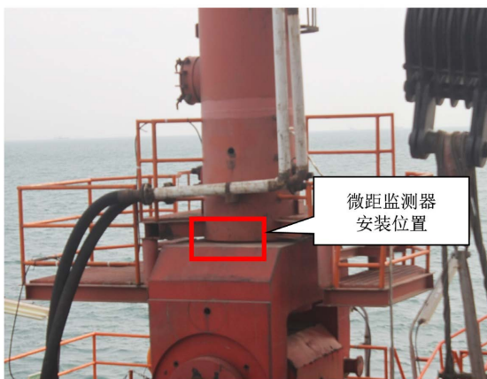
Figure 2. Customized function of single-point mooring monitoring system: mooring leg settlement monitoring
