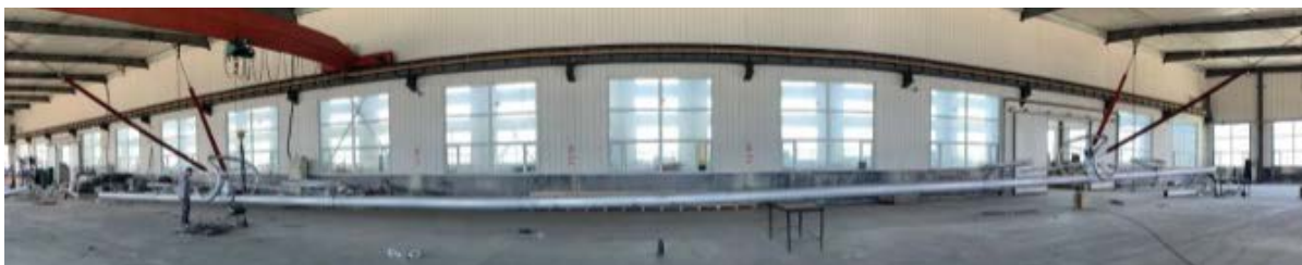
Figure 2. Photo of the tubular busbar tilted to one side
