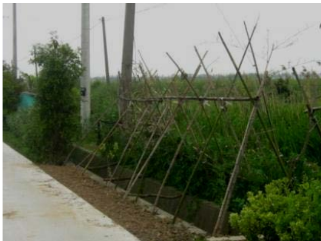
Figure 14. Damaged section of unnamed road in Maqiao village 图 14. 马桥村无名路被破坏的路段
