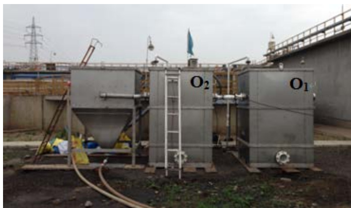
Figure 2. The pilot-scale IFAS facility
