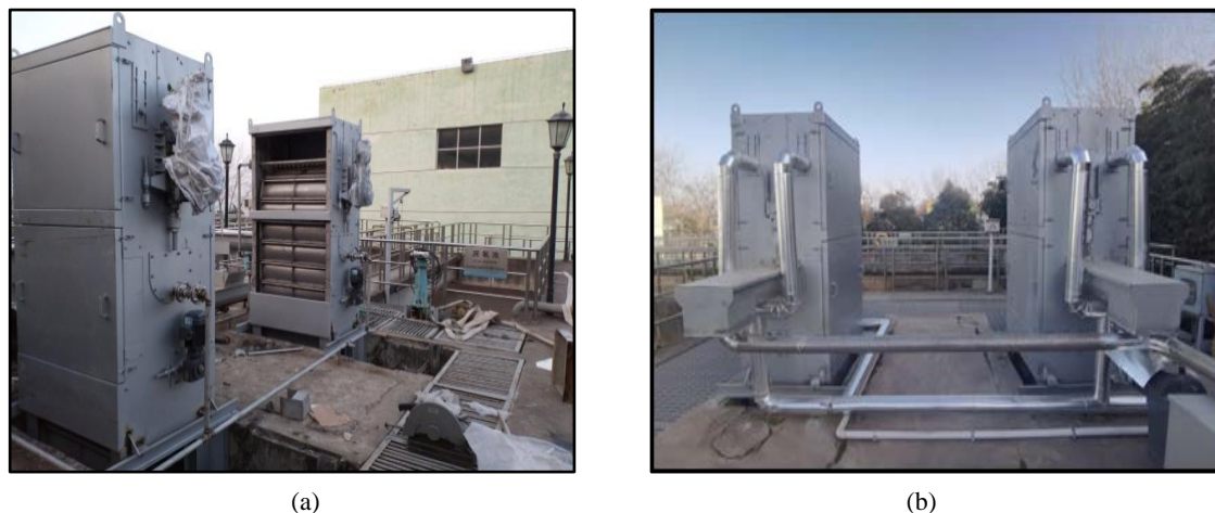
Figure 14. (a) Installing the internal runoff membrane grille; (b) The internal runoff membrane grille 图 14. (a) 安装内径流膜格栅; (b) 内径流膜格栅
