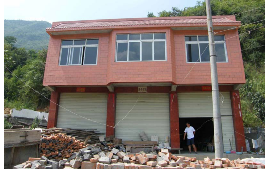
Photo 8. w6 windows and doors still can be freely opened, the bearing structure of no crack occurs, judged to be intact 照片 8. w6 门窗仍可以自由开启，承重结构没有出现裂缝，判断为完好结构
