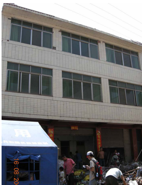
Photo 16. z10 doors and windows intact, visible horizontal cracks on the inner wall, judged to be medium damaged 照片 16. z10 门窗完好, 但内墙可见横向裂缝, 判定为中等破坏
