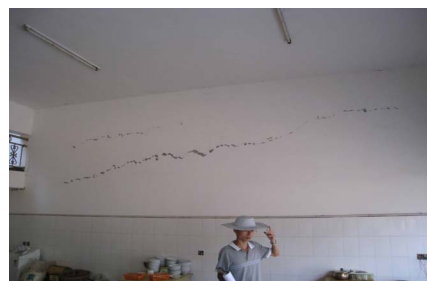
Photo 21. z35-1 the detail part of photo z35, horizontal cracks on bearing walls 照片 21. z35-1 z35 的细部图片, 可见承重墙出现水平贯通裂缝
