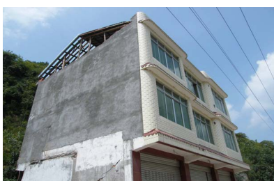
Photo 22. y17 overall structure slight tilt, large cracks on bearing walls, judged as serious damaged 照片 22. y17 整体有轻微倾斜，承重墙出现大裂缝，判定严重破坏
