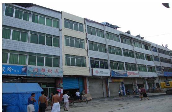
Photo 13. q14 cracks on bearing wall, judged to be slight damage building
