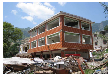
Photo 25. y39 columns in bottom tilted, judged as serious damaged 照片 25. y39 底层柱子倾斜方向不一，柱头损坏严重，判定为严重破坏
