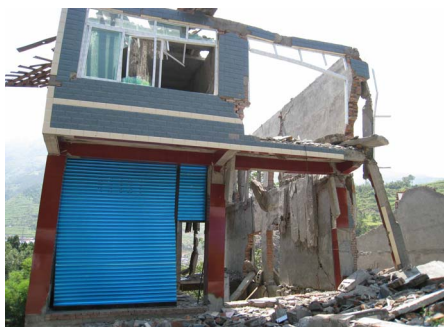
Photo 28. d17 most structural damage, beyond repair, judged as collapse 照片 28. d17 大部分结构构件损毁，无法修复，判定为倒塌
