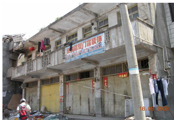
Photo 15. q40 structural integrity, the top is destroyed, judged to be slight damage building
