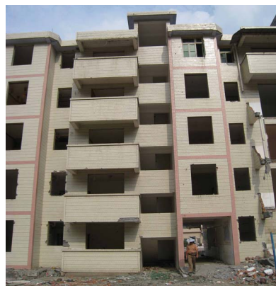
Photo 18. z20 structural integrity, the balcony seriously damaged x cracks on bearing walls, judged to be medium damaged 照片 18. z20 房屋结构完整, 但阳台损坏较严重, 承重墙出现 x 裂缝, 判定为中等破坏
