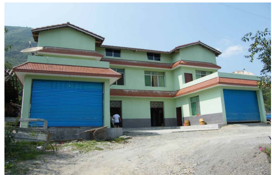
Photo 10. w7 a few frames of the window slight deformation, no large cracks, judged to be intact building 照片 10. w7 个别窗框有轻微变形，整体完好，无大的裂缝，判断为完好结构
