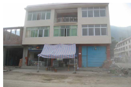
Photo 20. z35 structural integrity, doors and windows intact, but horizontal cracks on bearing walls, judged to be medium damaged 照片 20. z35 房屋整体结构完整, 门窗完好, 但内部承重墙出现水平向裂缝, 判定为中等破坏
