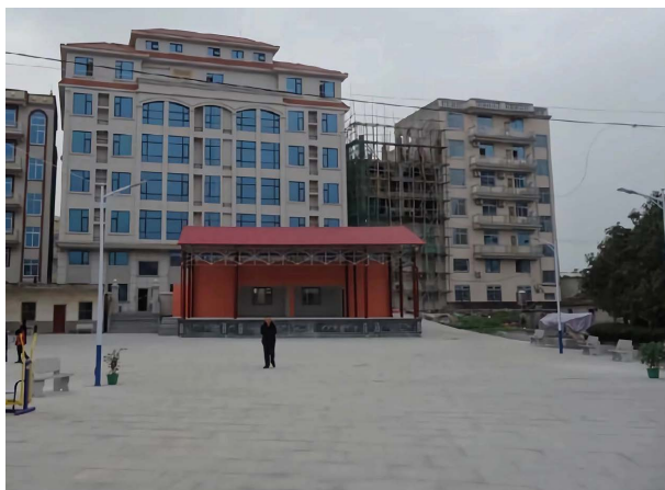
Figure 2. Construction of a large square in a village in Xianyou County 图 2. 仙游县某村修建大广场 ②
