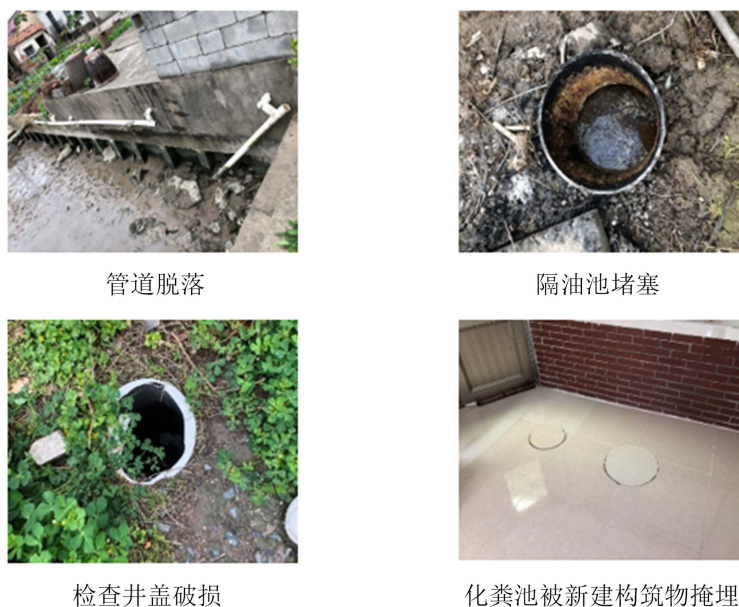
Figure 1. Sewage collection pipe network problem in Hengsha Township 图 1. 横沙乡污水收集管网问题
