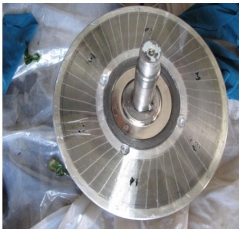
Figure 5. Scratches on rotor of submersible pump No.3
