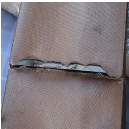
Figure 6. Discharge traces of low pressure side Magnetic shielding
