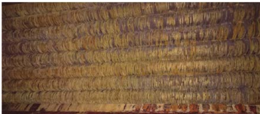
Figure 1. Abnormal scaling on the outer wall of economizer tube [10]
