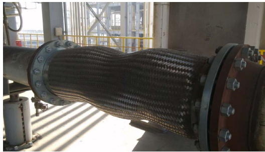
Figure 1. The using of the rinse water corrugated hose (Putting-in-service for 1 day)
