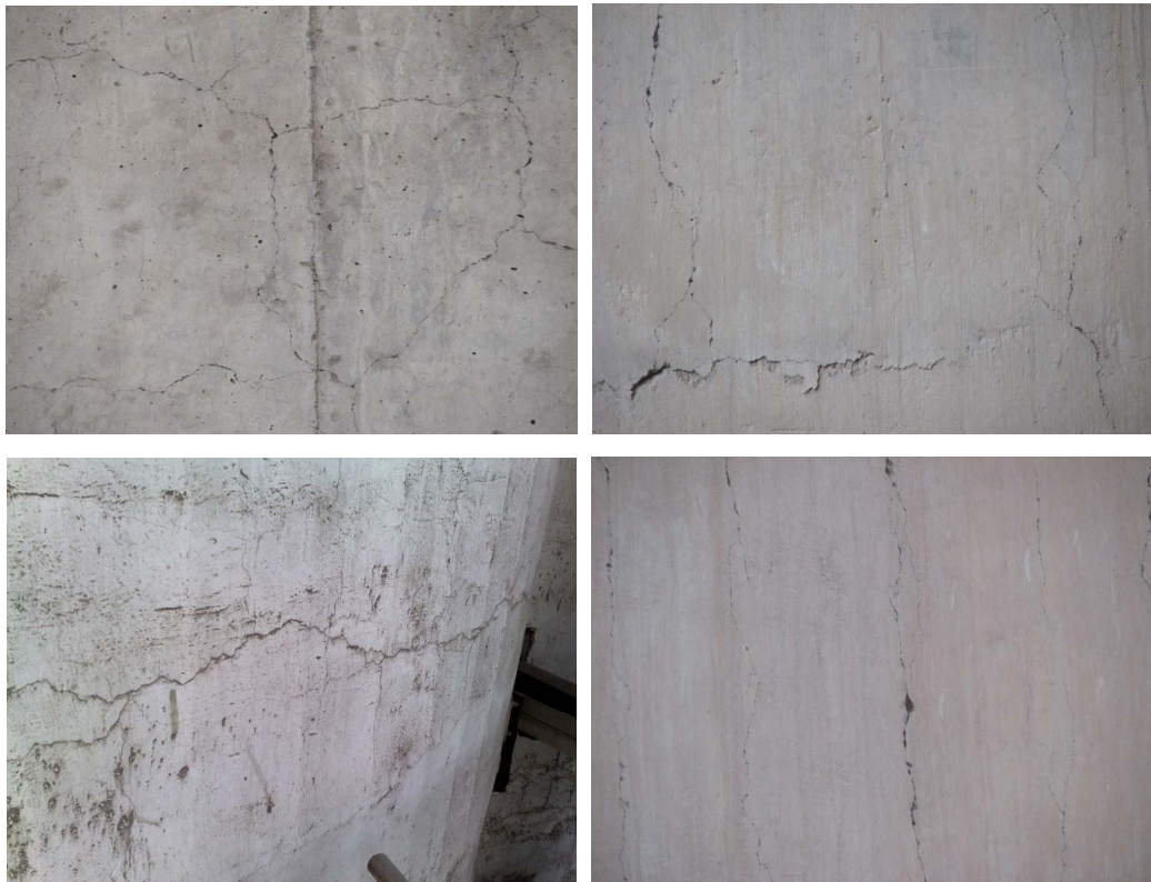
Figure 4. Annular and vertical cracks on reinforced concrete silos 图 4. 钢筋混凝土仓壁的环向水平裂缝与竖向裂缝
