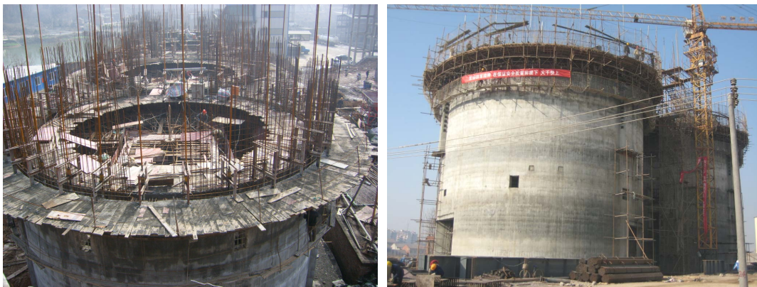
Figure 2. Slipforming construction of reinforced concrete silos 图 2. 钢筋混凝土筒仓滑模施工现场
