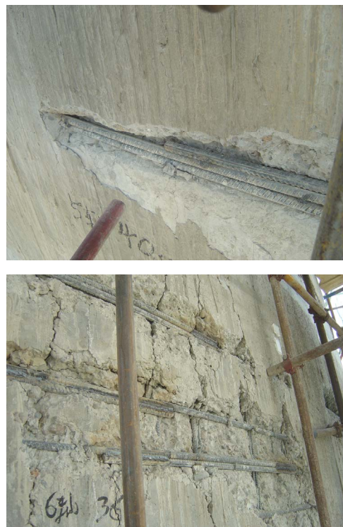
Figure 5. Visible colligated annular reinforcements in breakage region of concrete silo walls 图 5. 混凝土仓壁局部破损处外露的绑扎连接环向钢筋
