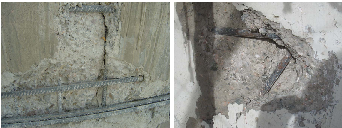
Figure 3. Visible reinforcements in breakage region of the concrete silo 图 3. 混凝土筒仓破损处的外露钢筋
