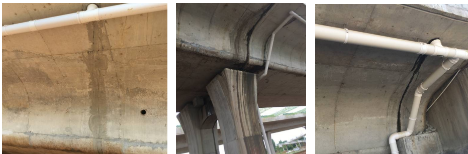
Figure 2. The watermark of bridge 图 2. 桥梁外观渍水图
