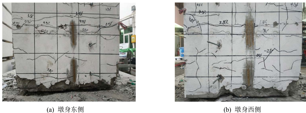
Figure 6. Failure modes of assembled pier specimen 图 6. 装配式桥墩试件破坏形态
