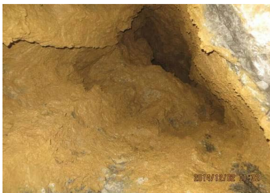
Figure 3. The Karst cavern located at Section DK308 + 120 of Caijiaguan Tunnel
