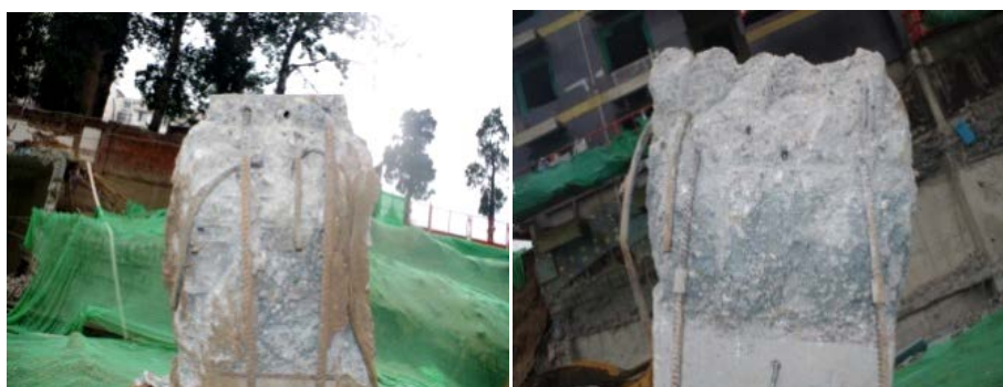
Figure 2. Top end of B1 story column after roof punching failure of the underground garage 图 2. 顶板冲切破坏后的负一层柱外露上端
