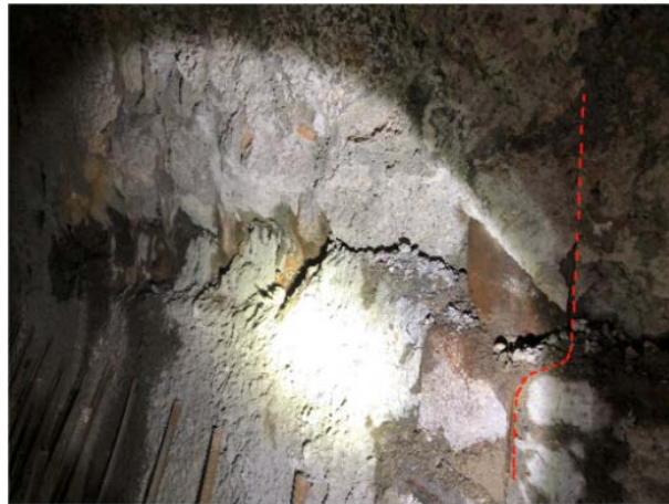
Figure 2. The buckling of the arch scaffolding on the right wall 图 2. 右边墙拱架弯折扭曲
