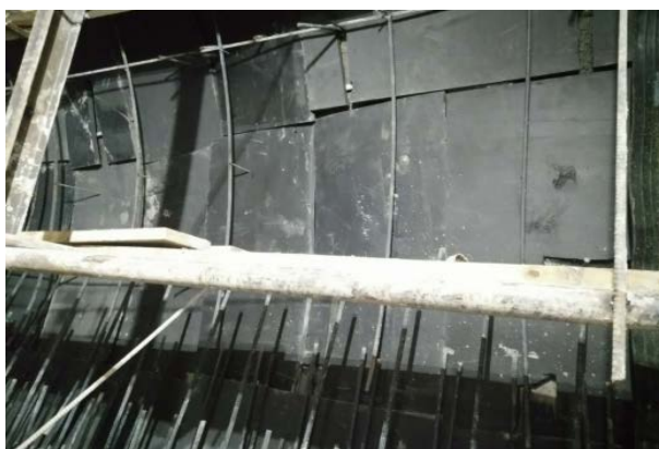
Figure 10. The side arch fixing on buffer layer in construction 图 10. 施工中缓冲层侧拱安装
