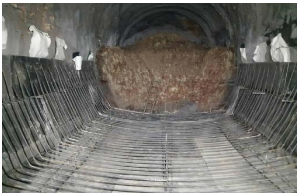
Figure 9. The inverted arch fixing on buffer layer in construction 图 9. 施工中缓冲层底拱安装
