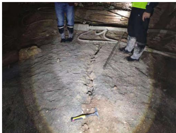
Figure 3. The bottom concrete cracks upward 图 3. 仰拱推土上抬开裂
