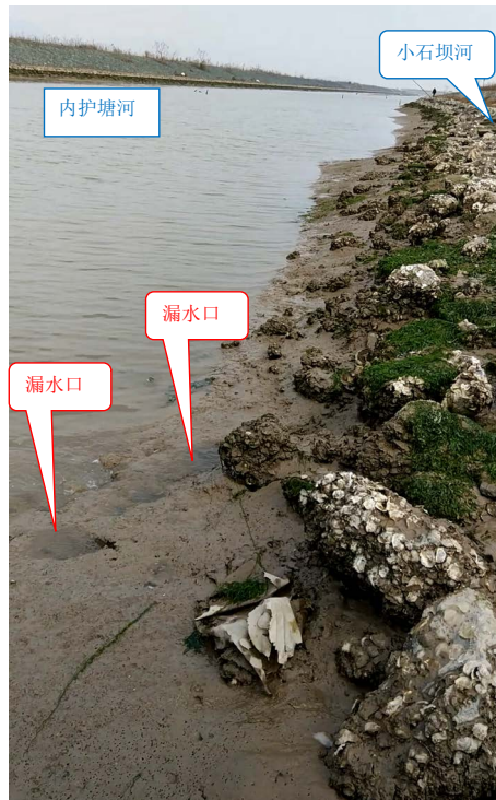
Figure 1. Current water leakage points 图 1. 现状漏水点
