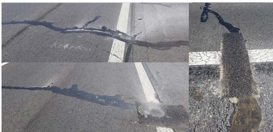
Figure 5. Reflection cracking and common treatment effect
