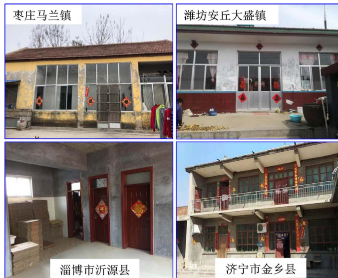
Figure 5. The problem of too large holes in vertical and horizontal walls of residential houses
