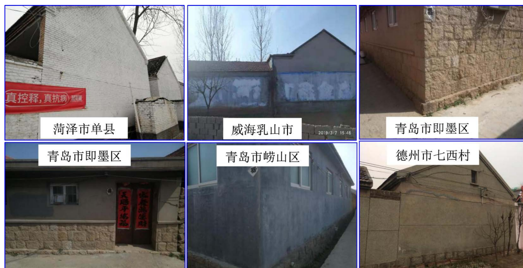
Figure 7. Insufficient seismic structural measures exist in residential buildings 图 7. 民居存在抗震构造措施不足问题
