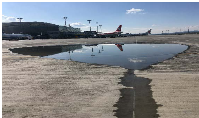
Figure 2. Ponding after rain in subsidence area of the isolation apron 图 2. 隔离机位沉陷区雨后积水情况
