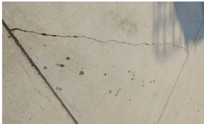
Figure 5. Broken cement pavement plate of the isolation apron 图 5. 隔离机位水泥道面板块断板
