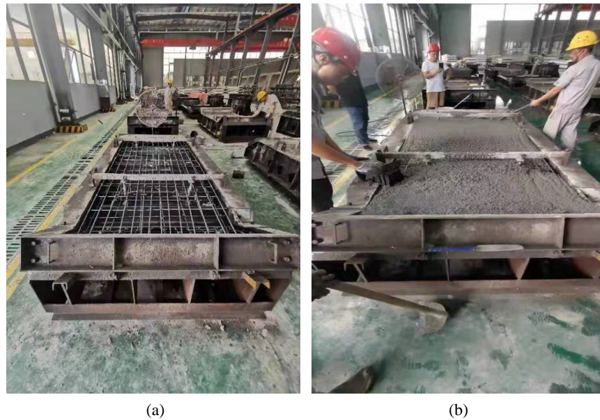
Figure 4. Precast staircase factory processing. (a) Stair mold and reinforcement situation; (b) Stair concrete casting situation
