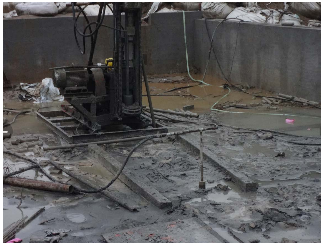
Figure 3. Construction pictures of high-pressure pile tip grouting 图 3. 高压桩端压浆施工图片
